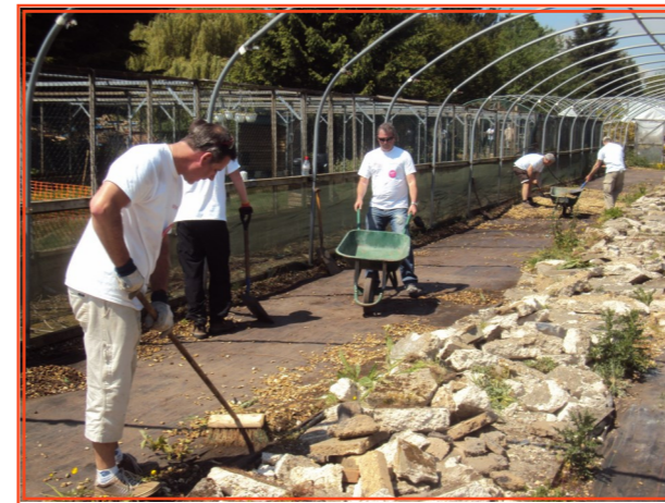
The Arqiva Company Busy on the 'Give and Gain Day' in May. Clearing the way for the play area in The Seedlings centre.
